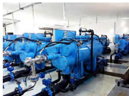
Gostivar water supply system – mechanical microfiltration (North Macedonia)
