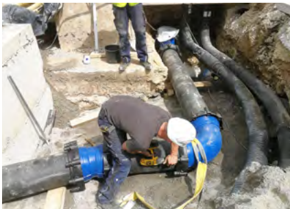
FM certified ductile pipes for the sprinkler system in the BSH company in Nazarje (Slovenia)
