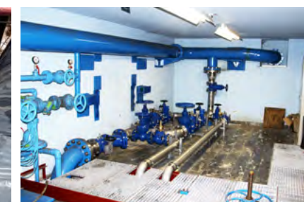
Zadlaščica pressure reducing station, 43-11 bar (Slovenia)
