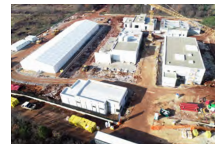
Central waste water treatment plant in Poreč (Croatia)
