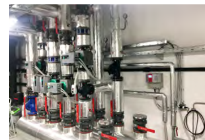
Ultrasound flow and temperature meter for the Cargo Partner company (Slovenia)
