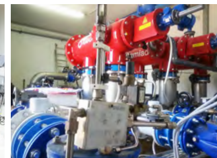
Irrigation system Kalce-Naklo, Municipality of Krško (Slovenia)
