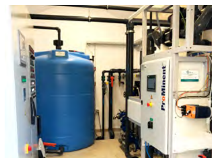
Drinking water treatment plant in the Podstenjšek waterworks – ultrafiltration (Slovenia)
