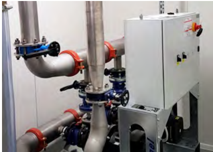
Manifold system for cooling of industrial water in the TEM Čatež company (Slovenia)
