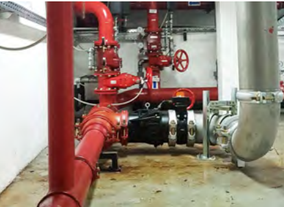
Fire safety system in the Krka company (Slovenia)
