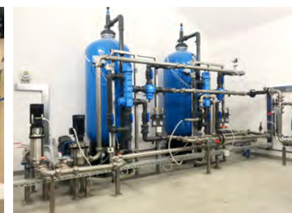
Drinking water treatment plant in Podslivnica – sand filtration (Slovenia)
