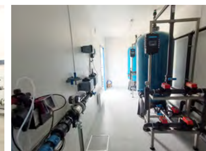
Sand filtration for drinking water - container version, Đulovac (Croatia)
