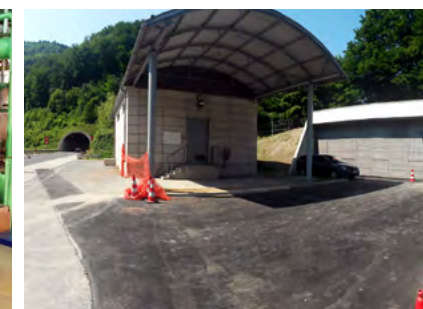
Fire hydrant network in the Ločica tunnel with pumping station in compliance with the VdS standard (Slovenia)
