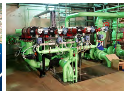
Cold water filtration in the TE-TOL Ljubljana power station (Slovenia)
