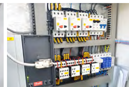
Installation of a SCADA system for WC-BIT 3 (North Macedonia)
