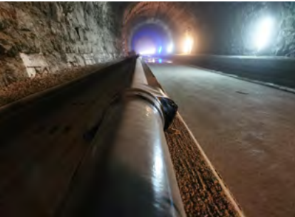
Hydrant network of the Karawanks Railway Tunnel (Slovenia)
