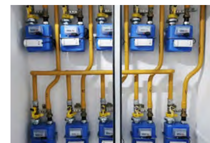
Remote reading of gas meters and remote monitoring for key customers LoRaWAN, GSM, NBIoT for Dukom Plin, Dugo Selo (Croatia)
