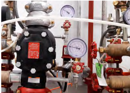
Sprinkler systems in the Navigator Business Centre in Belgrade (Serbia)
